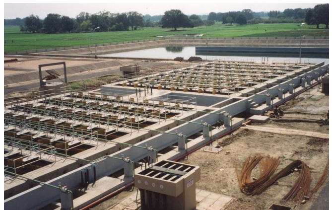
Top view of Mirzapur UASB plant. The UASB reactors are located largely underground.
